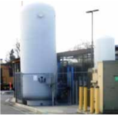
New Accumulation Tank on Main Compressors
